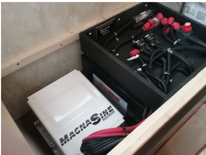
2800 Watt Inverter with 3 200AH batteries
